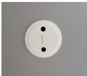
Occupancy counter camera
